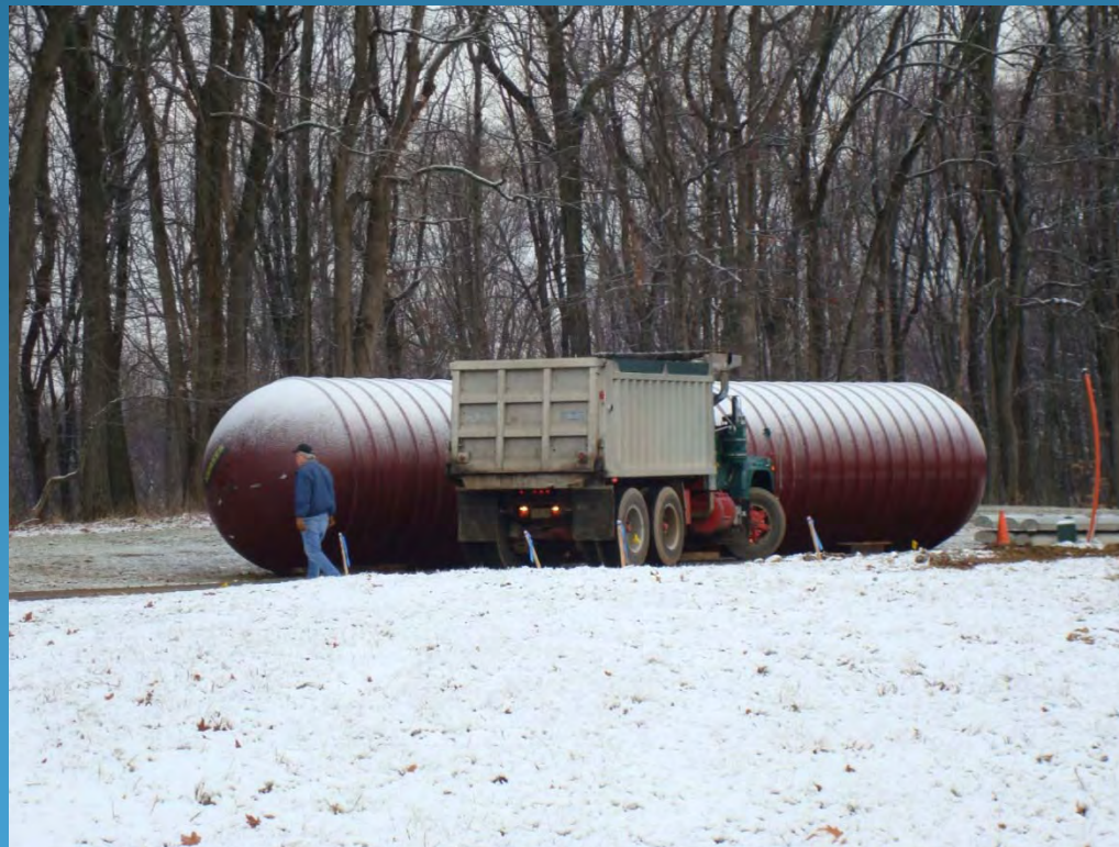
INSTALLATION FOR FIRE SUPPRESSION- MENDHAM, NJ
