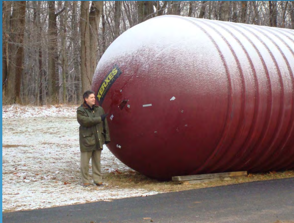
INSTALLATION FOR FIRE SUPPRESSION- MENDHAM, NJ
